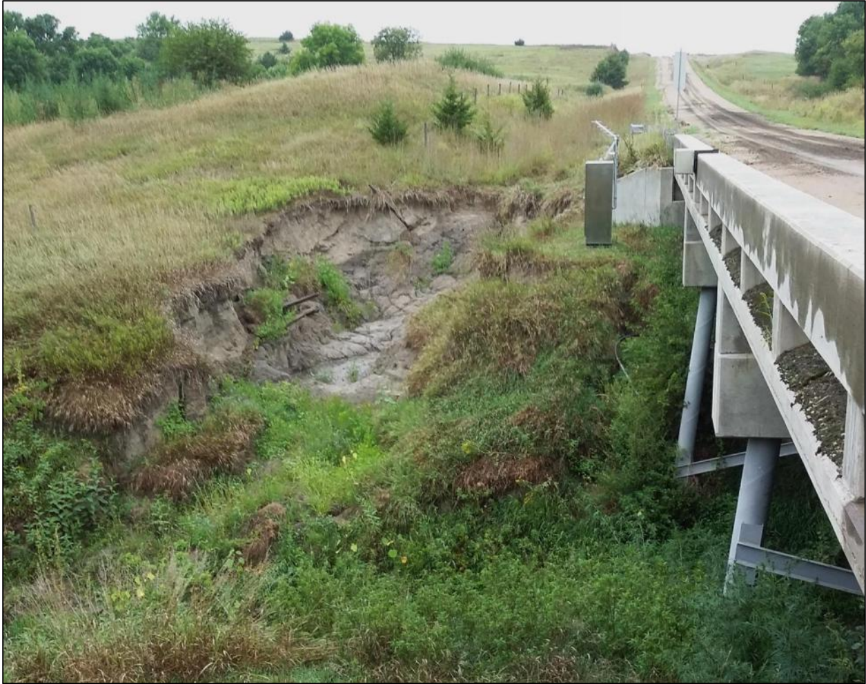
Figure 9. View west showing saturation slump threatening gage at Rd 726.
